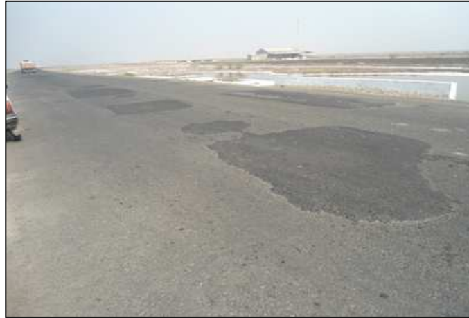
Fig – 3 Failure of Recently constructed Pavement after Monsoon due to High Swelling
